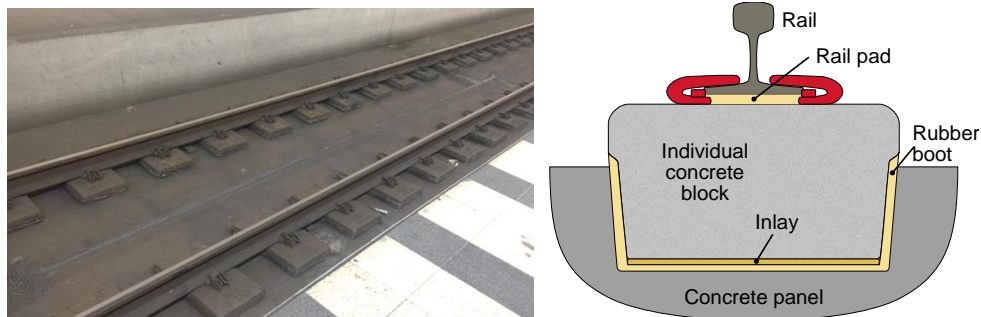
Figure 3. Left: Track with booted sleepers in Malmö, right: construction of the sleeper and boot.
